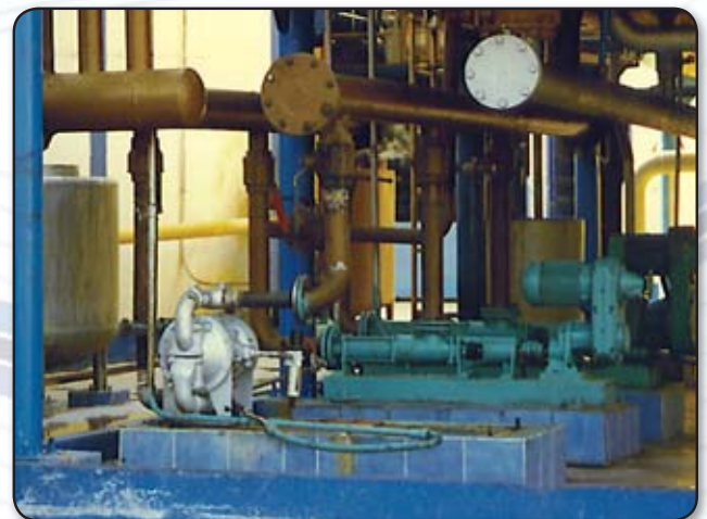
Solution providing AODD pump installation selected to reduce total costs of ownership and minimize floor space allocation.
