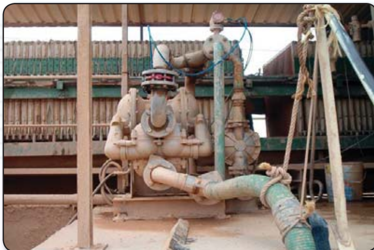
3" HDB bottom ported pump installed as a plate & frame filter press, pre-coat supply pump.
