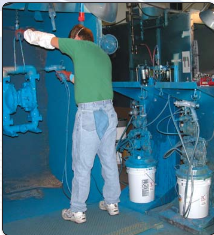
Pail mounted SANDPIPER® Pumps installed on paint spray booth station.
