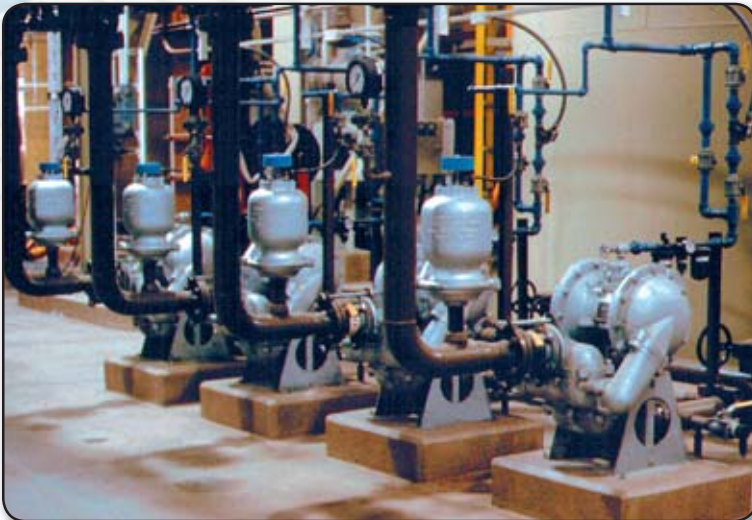
HDB bottom discharge ported pumps with tranquilizers installed at an industrial waste treatment facility.
