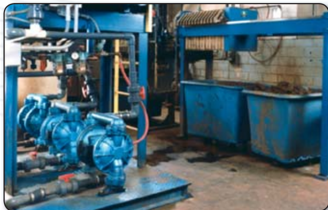
Metallic standard duty pumps handling suspended solids in an industrial waste treatment operation.
