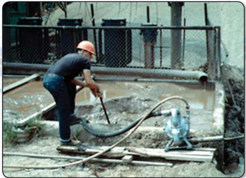
Heavy duty flap valve pump temporarily installed pumping settling pond sludge. (Perfect alignment not required).
